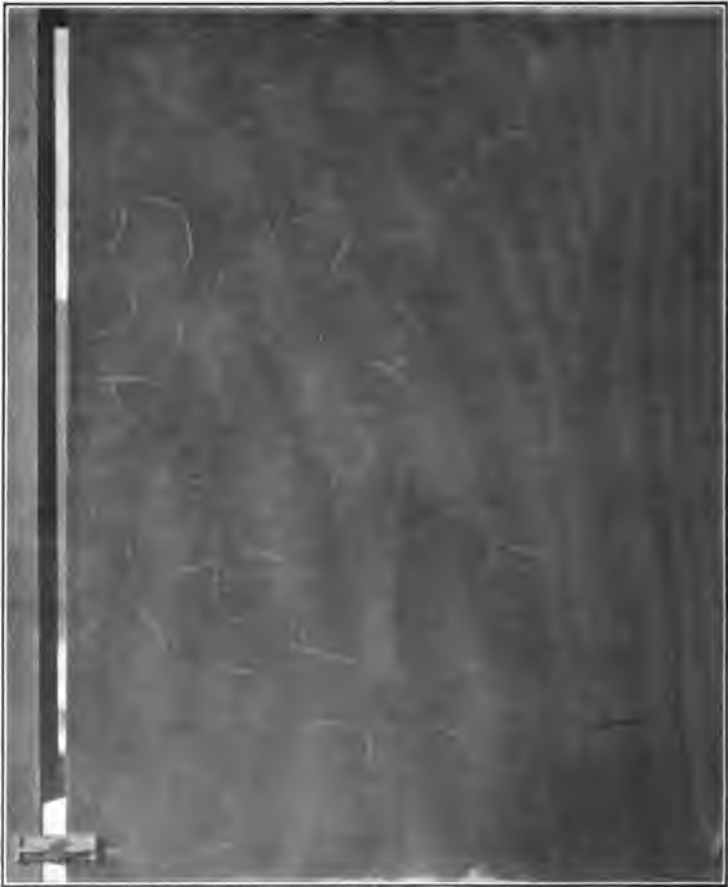
FIG. 66. — Alligatoring of coal tar over red lead.
